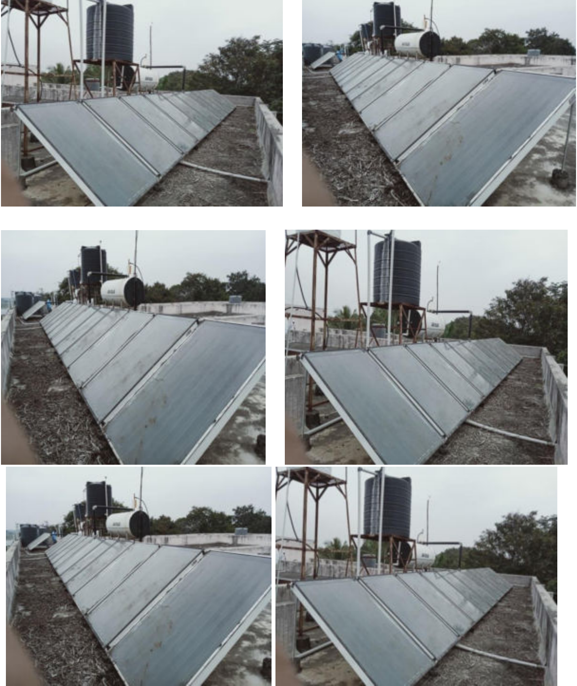
*Solar Energy Plant for Hot Water System in Ladies Hostel
