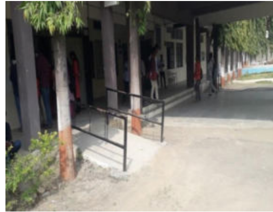
Ramps for Divyangjan
